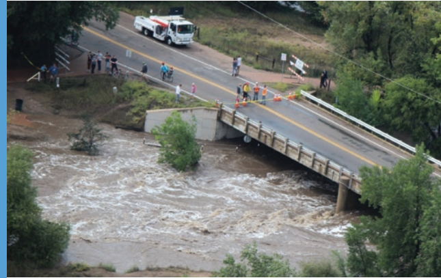
Poudre River flooding at Shields Street bridge
