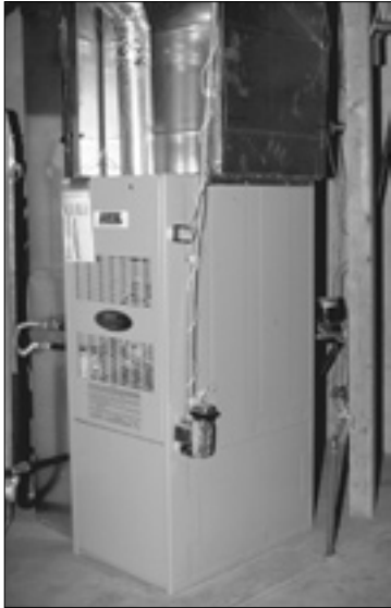
Induced-draft furnaces supplied space heating in almost all study homes.
