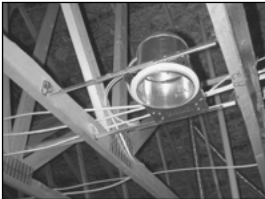
“Airtight” cans for recessed lighting reduced air leakage through insulated ceilings.
