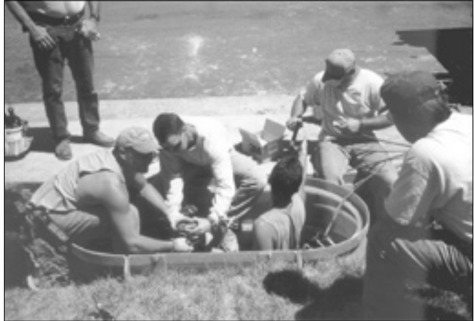
Fort Collins Utilities crew members change out a transformer that was overloaded under peak summer demand conditions.
