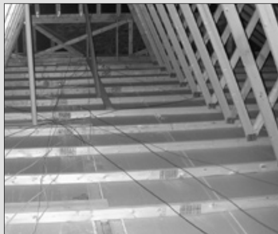
Several months after occupancy: no insulation in the attic.
