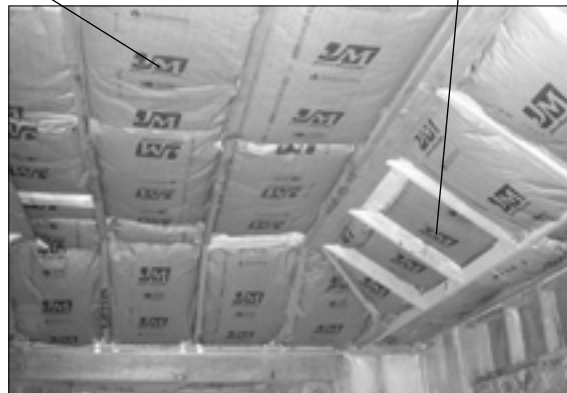
Vaulted and cathedral ceilings tended to have more insulation installation problems than flat ceilings.
