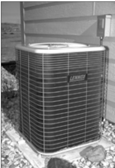
About half the study homes had central air conditioning. The compressor and condenser were located in an outdoor unit like this, with the expansion valve and evaporator coil located in the supply plenum at the furnace.
