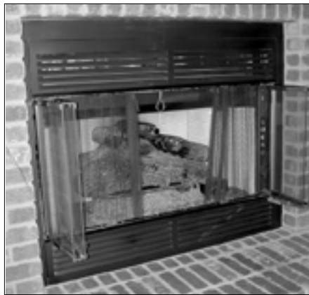
The flue, draft hood and outdoor air supply all contributed to leakage through atmospherically vented fireplaces.
