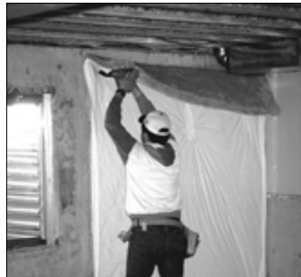
Basement wall insulation addressed one of the biggest remaining heat loss paths. The typical approach was a vinyl-faced fiberglass blanket on the interior of the concrete foundation.
