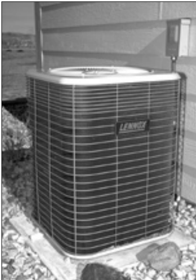
Outdoor air conditioning unit
