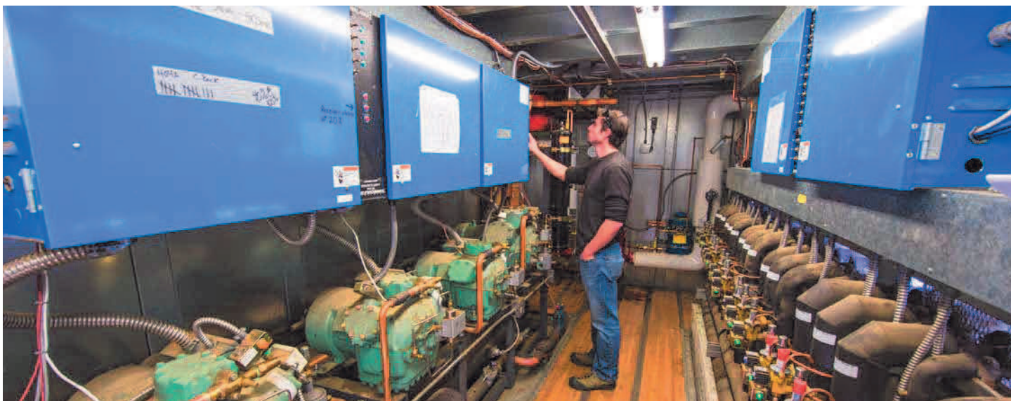
An NREL engineer checks the operation of the refrigeration system. Photo by Dennis Schroeder, NREL.
