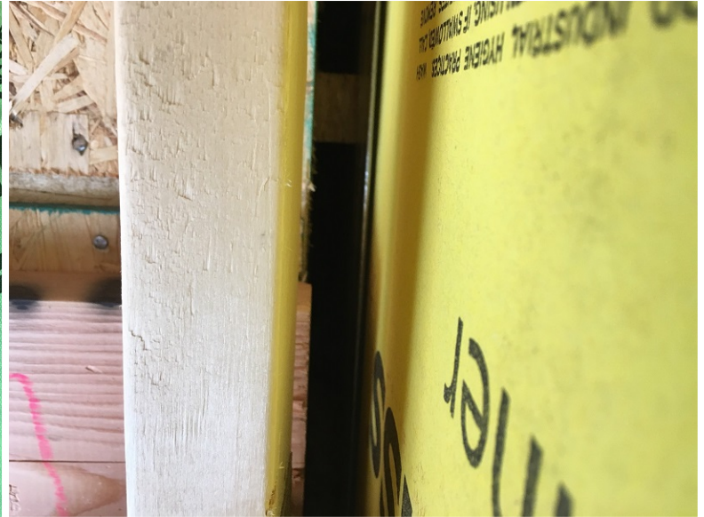
Gap between sheathing & shaftliner allowing air behind rim.
