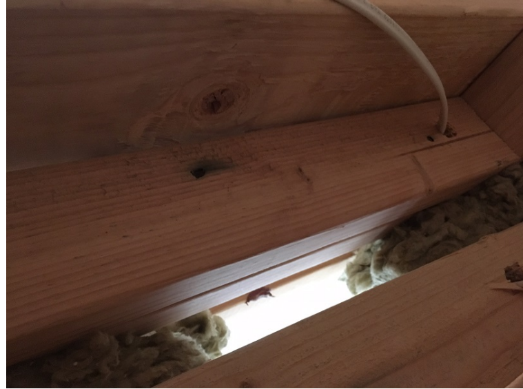
Looking down from above. Chinking removed shows direct connection with attic.
