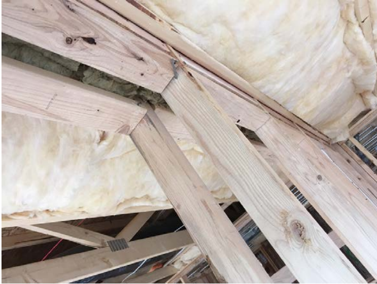
Looking up at top plate – gap chinked with mineral wool for draft stop.
