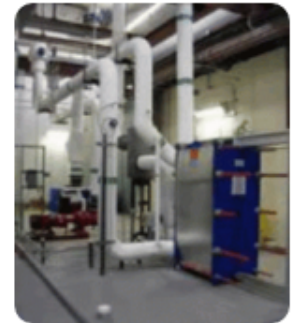
This free-cooling heat exchanger system reduces electricity bills by over $40,000 per year.
