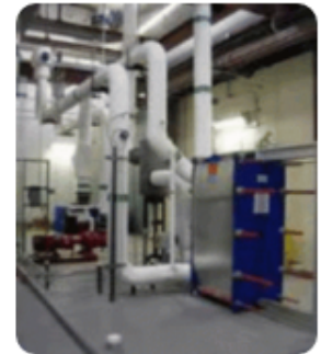
This free-cooling heat exchanger system reduces electricity bills by over $40,000 per year.
