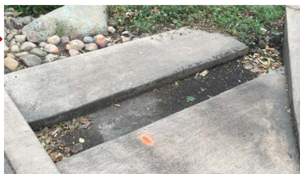
Presettling forebay example at Library Park
