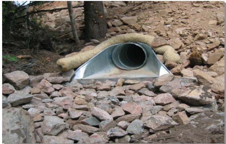
Photograph TOP-1. Riprap outlet protection.
