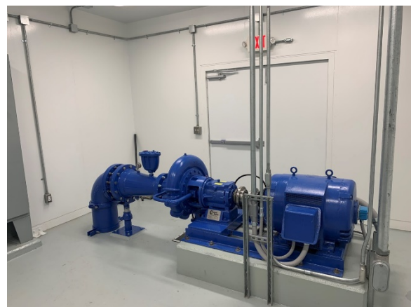
Figure 1. The Microhydro Generator
