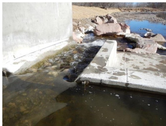
Figure 5.12: Recently installed fish passageway at the Fossil Creek Inlet Ditch just downstream of Prospect Avenue.
