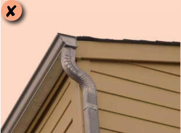
Figure 166: This eave is inappropriate because it does not provide an overhang.
