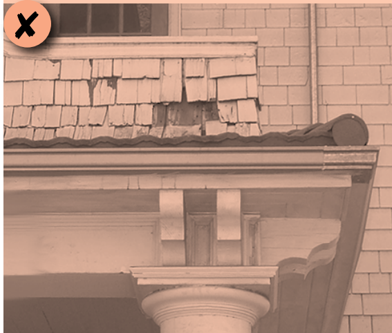
Figure 68: Do not remove damaged materials that can be repaired. In this case, loose shingles may be re-secured while missing ones may be replaced.
