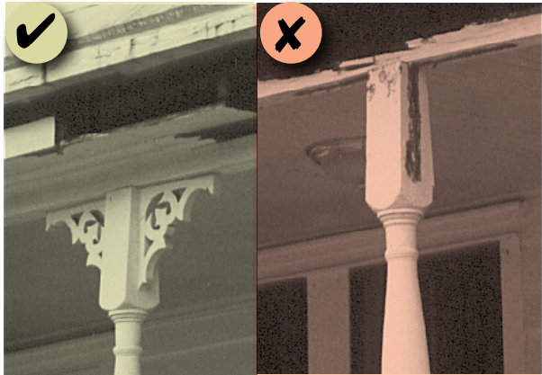
Figure 72: Replace missing original details in kind.
