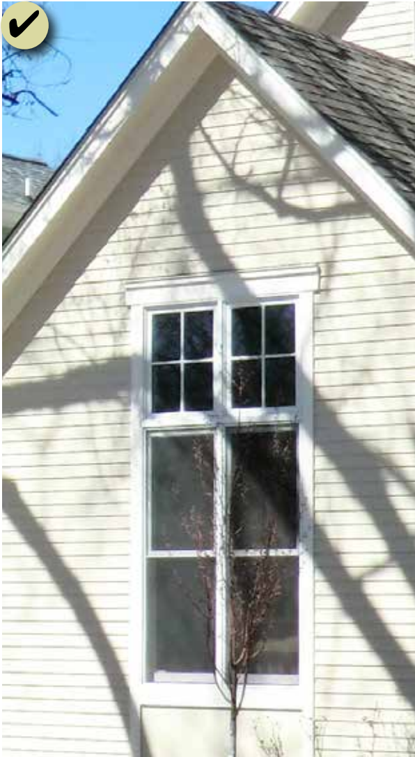
Figure 156: Use window and door widths, heights and materials that are similar to doors on historic buildings in the surrounding historic context.
