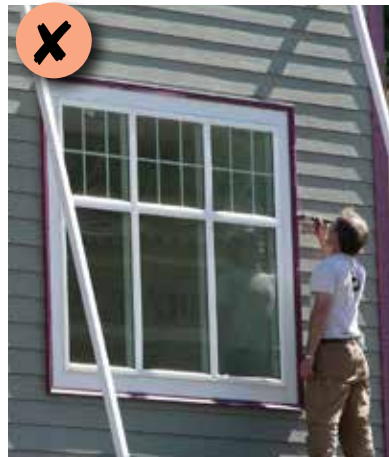
Figure 85: The windows and siding have both been inappropriately replaced with vinyl.
