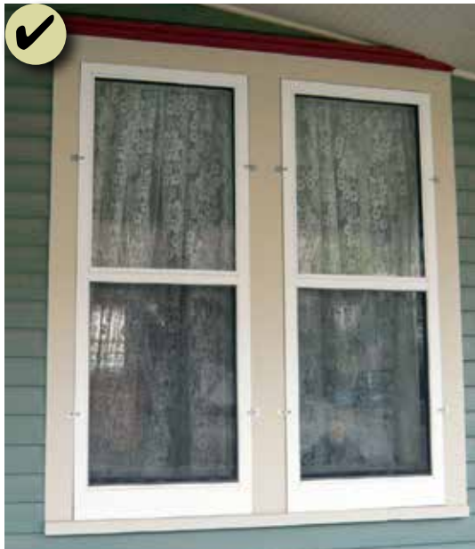
Figure 90: The storm windows match the opening; however, it would be more appropriate if the frames were wood to match the original material.
