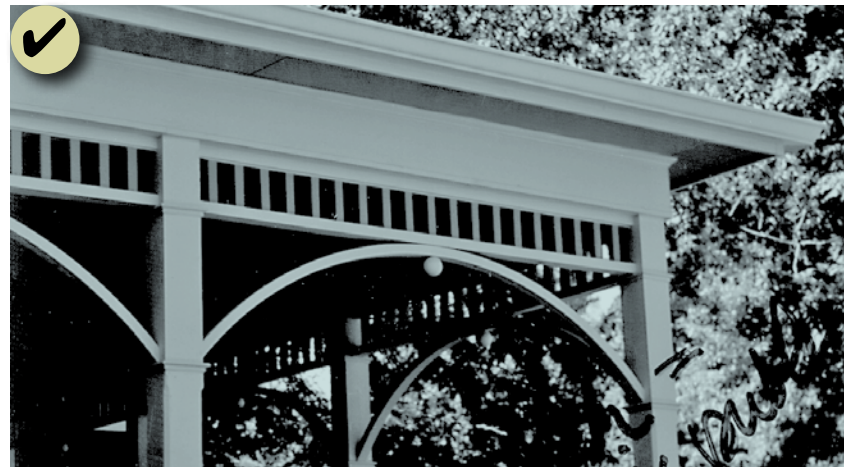
Figure 74: When reconstruction of a historic feature is impossible, develop a new design that is a simplified interpretation of it. This detail in the porch bracketing has simple vertical and horizontal elements rather than the historic curvature detail.
