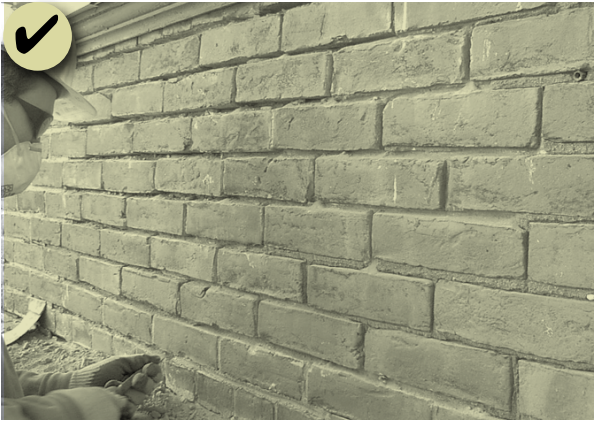
Figure 75: Re-point mortar joints where there is evidence of deterioration. Use correct mortar to prevent problems and match the historic design.
