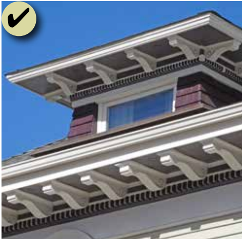
Figure 63: Maintain significant character-defining features, including: projecting cornices, decorative moldings and brackets and dentils and shingle siding at dormers.
