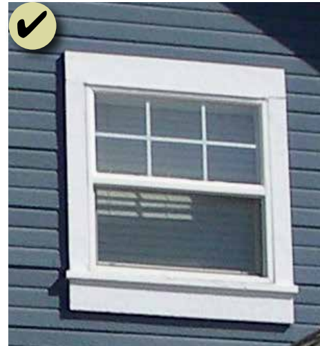
Figure 160: Set back a window or door from the outside wall plane so a reveal is evident, resulting in a shadow line around the opening.
