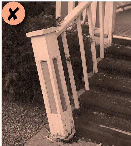
Figure 70: Before: A deteriorated railing should be repaired, not replaced, when feasible.
