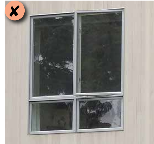
Figure 157: Design windows, doors and other features to be compatible with the historic context.
