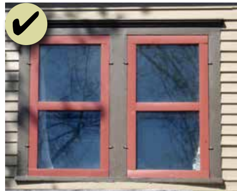
Figure 91: The storm windows match the opening; however, it would be more appropriate if the frames matched the historic window sash similar to the image shown above.
