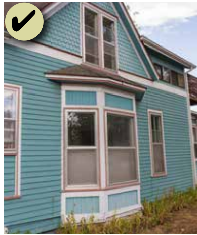
Figure 81: Preserve historic window features including the frame, sash, muntins, mullions, moldings, glazing, sills, heads, jambs and groupings.
