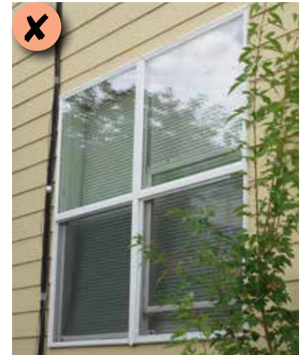
Figure 161: A window should not appear flush with the outside wall plane.
