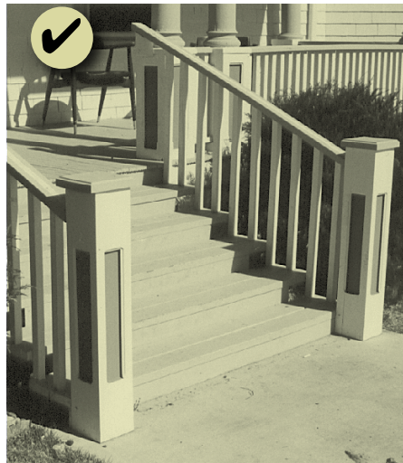
Figure 71: After: Railing has been repaired and the base of the post has been replaced in-kind. This is an appropriate approach.
