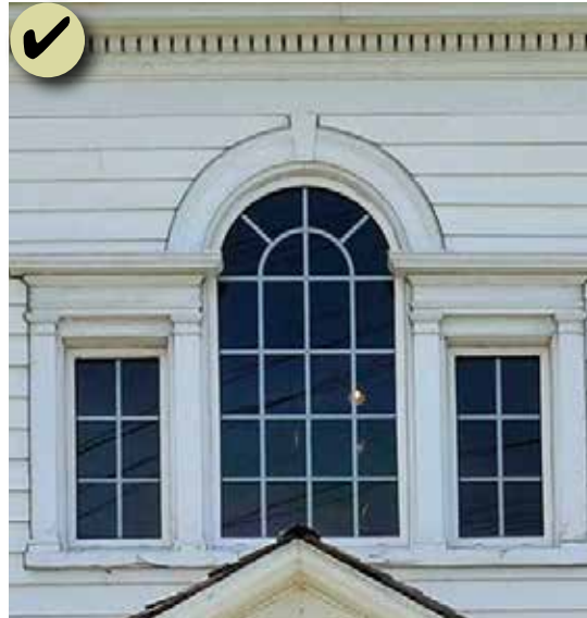
Figure 64: This palladian window with wood tracery is a character-defining feature that helps to convey the building's architectural style and should be preserved.
