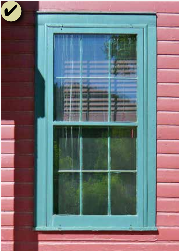
Figure 123: Consider using a storm window to enhance the energy efficiency of an existing historic window, rather than replacing it.
