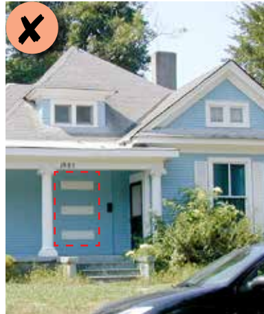
Figure 84: This three pane window alteration is inappropriate and should be restored to its original historic configuration.
