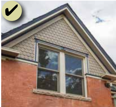
Figure 83: Roof overhangs and eave details are important to maintain the character of the building.
