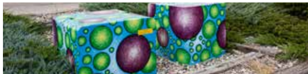
46 painted transformer cabinets
