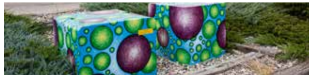
46 painted transformer cabinets
