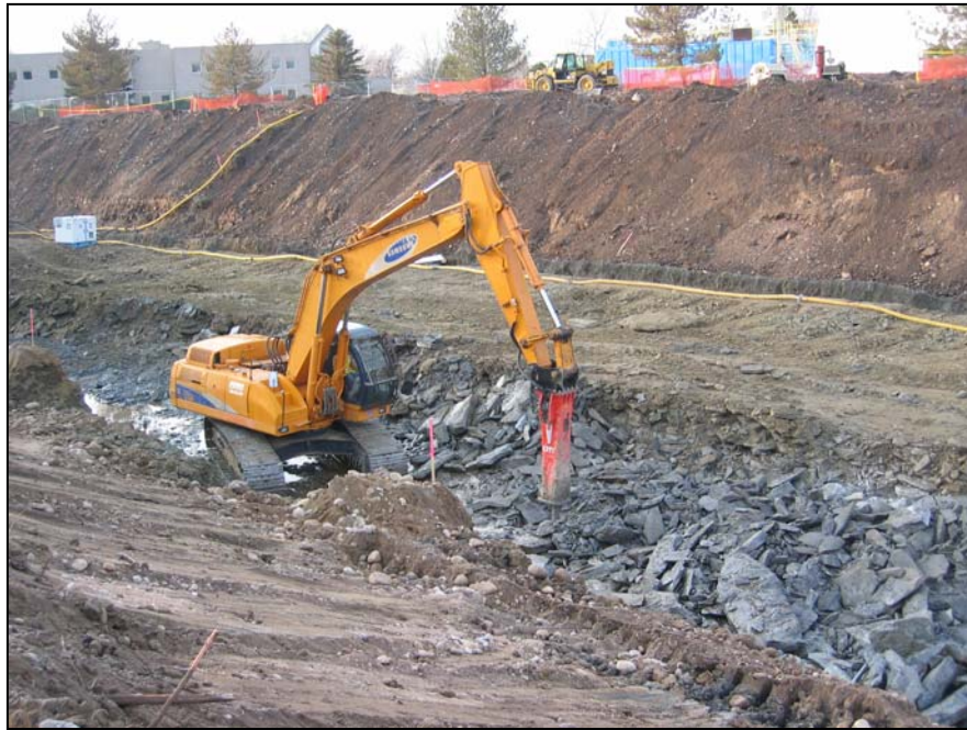
Photo of breaker equipment used to remove contaminated bedrock from river bed.
