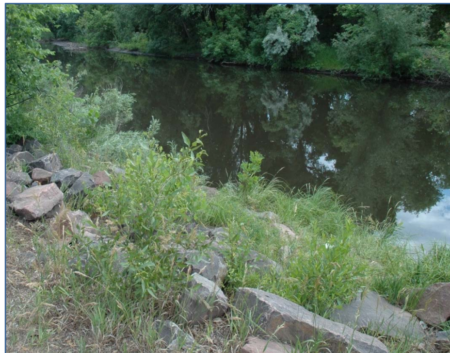
Figure 2.20 Exposed Riprap on the North Bank at Legacy Park
