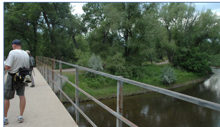
Figure 2.11 McMurry Pedestrian Bridge, Note Non-Compliant Railing
