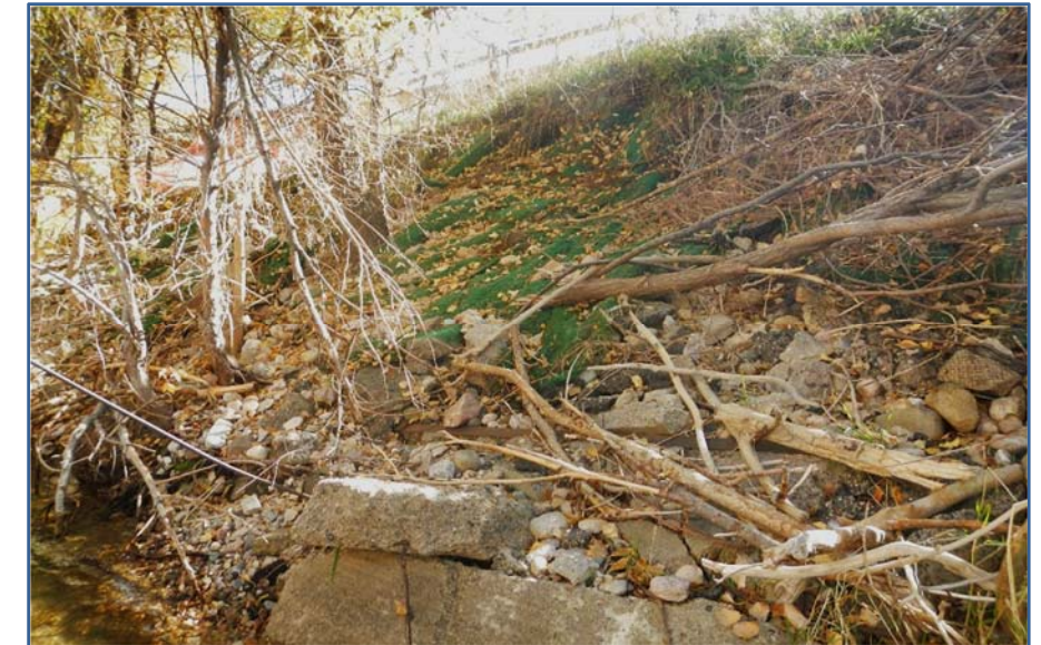
Figure 2.35 Bank Erosion, Concrete Rubble, and Exposed Plastic Turf Mat on South Bank, West of the BNSF Railroad
