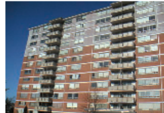
Photo 3: Exposed Frame. The bad news is that we have built lots of these. The good news is that they are easy to fix by recladding them with exterior insulation.
