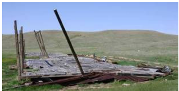
Collapsed pole barn near Brannigan Springs
