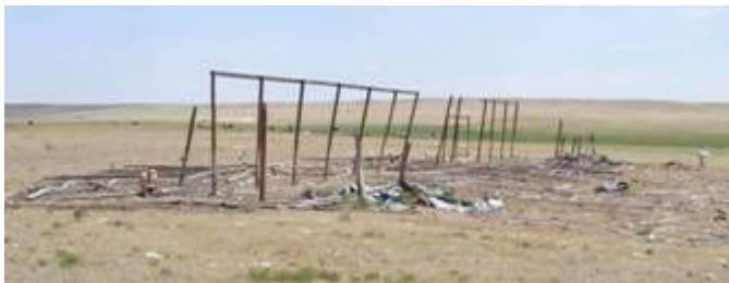
Collapsed livestock building at Jack Springs Camp
