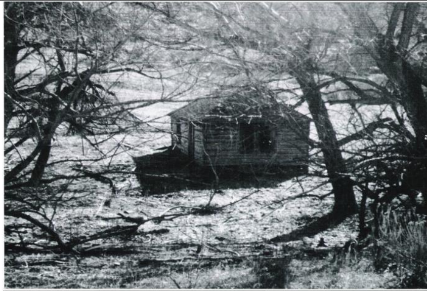
Recent years photo before roof collapse
