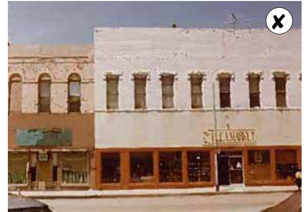
Interim image of missing cornice.
