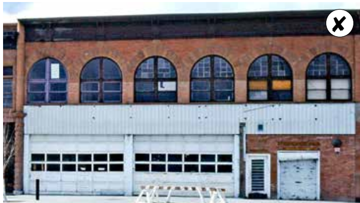
Before rehabilitation: upper story windows in need of repair.
