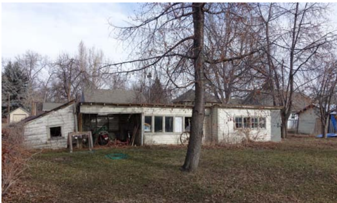
Figure 4-14: Chicken coop behind house at 117 N. Whitcomb, one of many such outbuildings built in the Loomis Addition (Mary Humstone, 2015).
