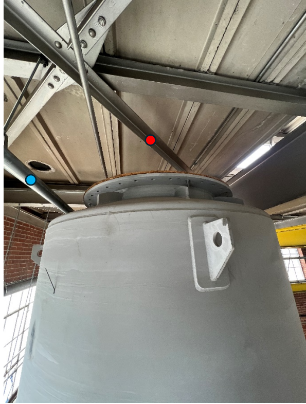
Fig 4. Photo of silencer at ceiling
