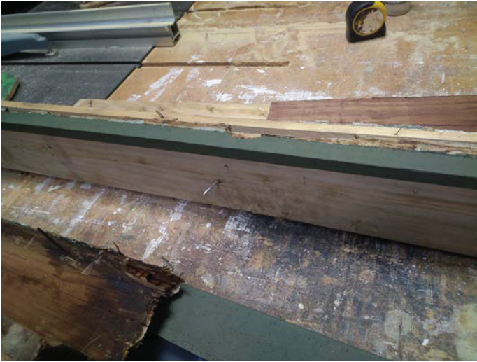
Figure 2: Failed Sill with galvanized nails
