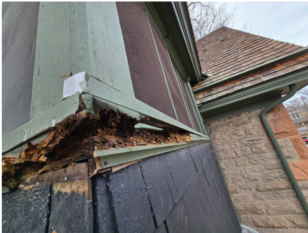
Figure 1: Rotten Sill showing tin cover.
