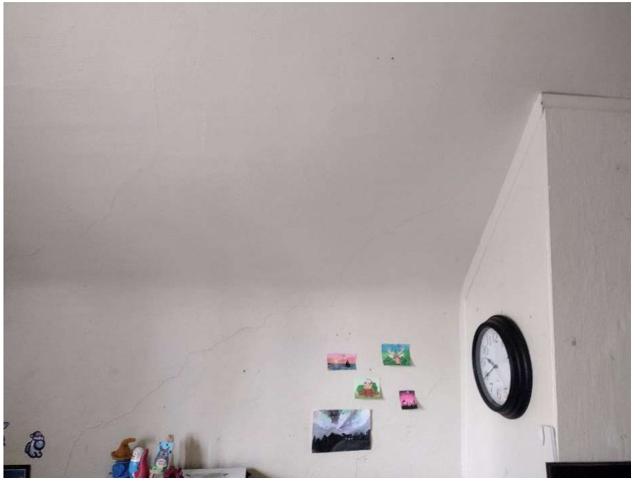
Figure 1: Cracking in Walls - North Bedroom at Second Floor
