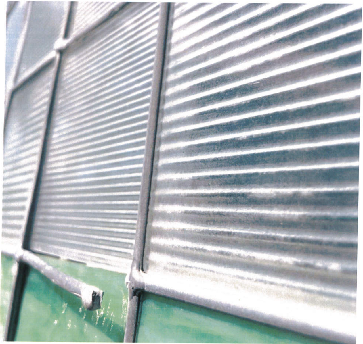
Solder joints are splitting under pressure from warping and age.
