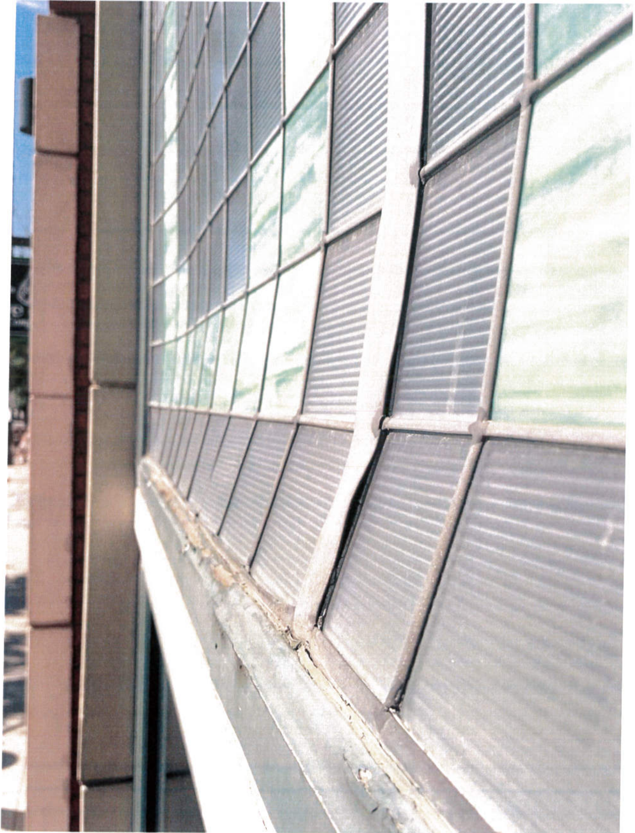
Zinc caming is warping (buckling), causing a wavy appearance.
