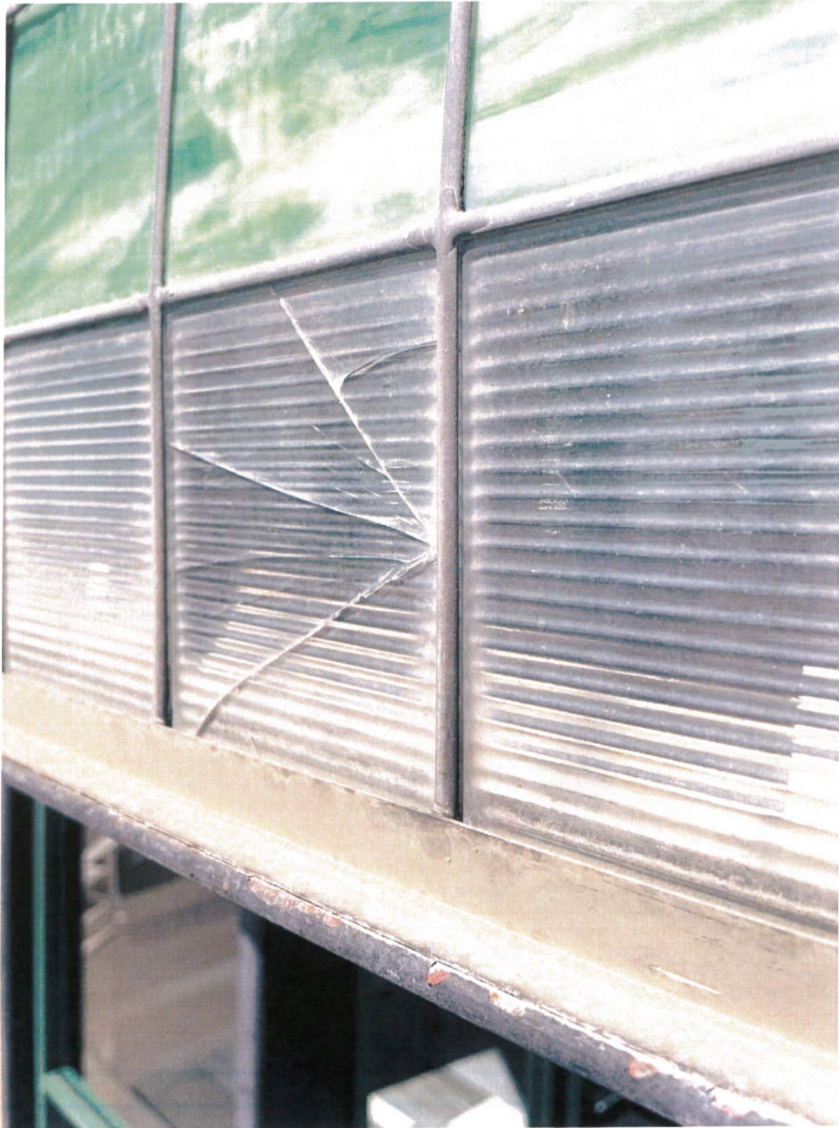
Broken glass due to warping, harsh weather, vandalism, and accidental damage.
