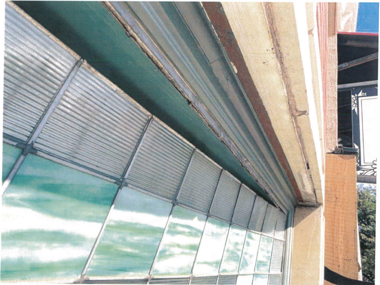
The glass has separated from the outer zinc edging at the top.
