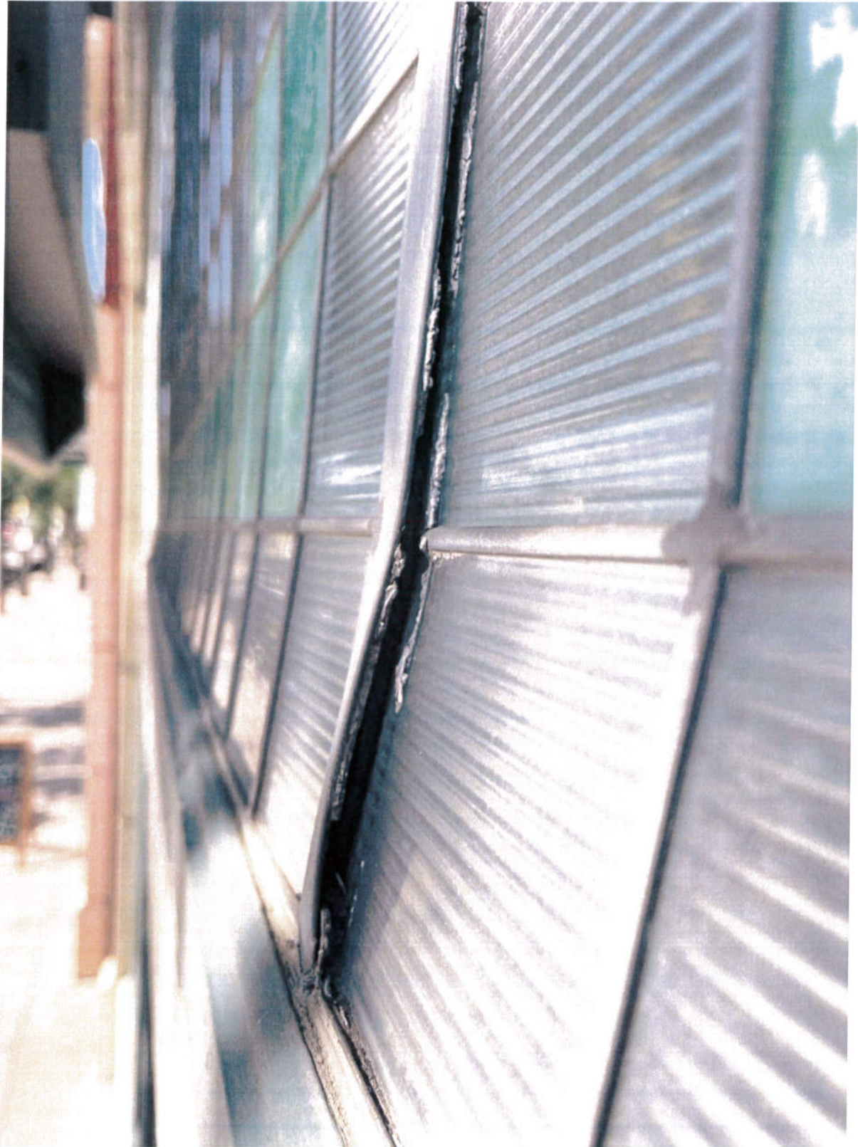
Zinc/ glass separating in places exposing the interior.
