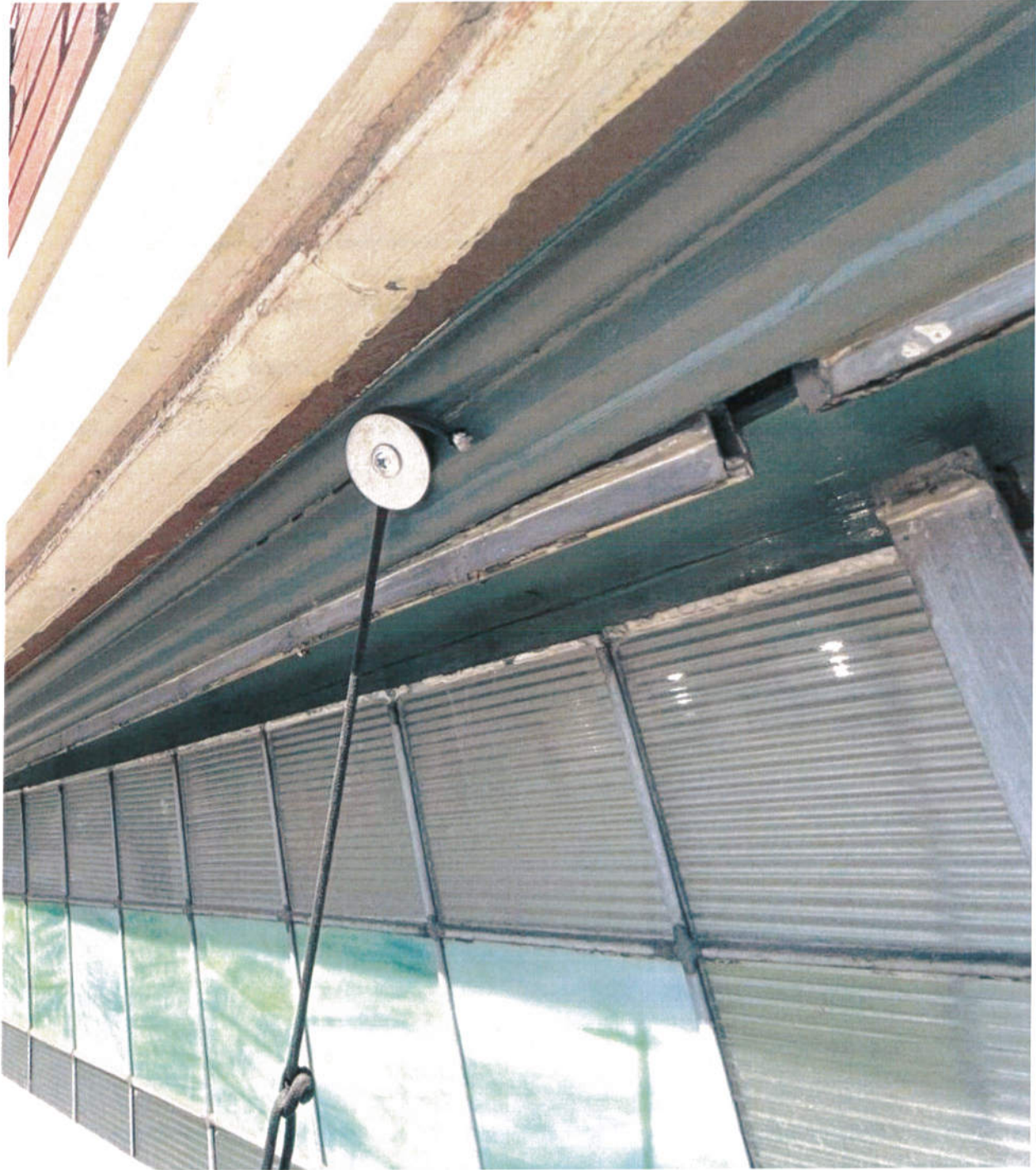
Rebar is separating from stained glass and dislodging from frame.
