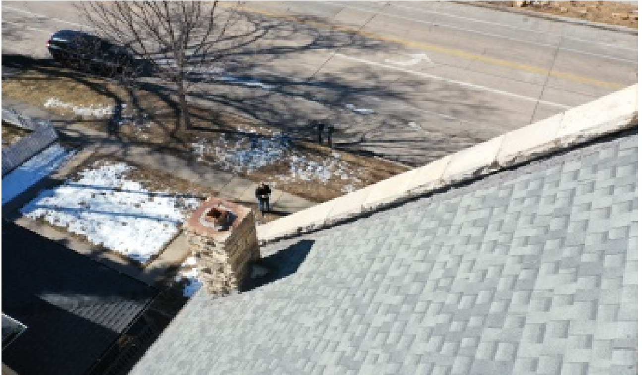
Figure 4: Roof showing existing tar flash of roof to parapet. Note chimney flash.
