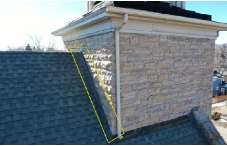
Figure 2: Yellow box showing roof - wall flashing failure. Flashing at top of roof and wall meeting looks to be holding but missing counterflashing.
