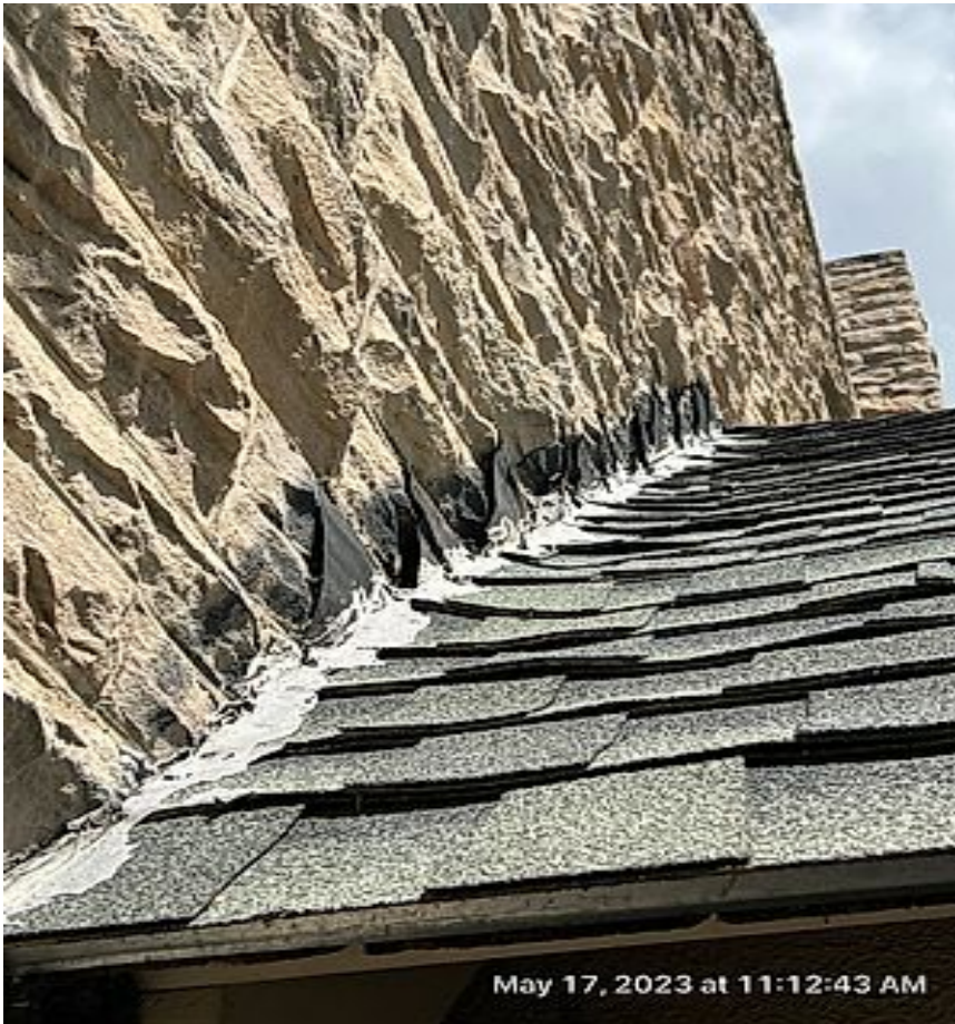
Figure 1: Existing conditions - Tall wall to roofing. Note some reglet flashing installed.
