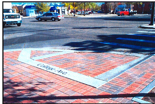
EXISTING OLD TOWN RAMP SHOWING PAVING PATTERN, CONCRETE WORK AND STREET NAME
