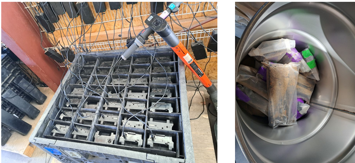
Figure 8. Batteries in the charging array (left) and packed in flame retardant for disposal (right)
