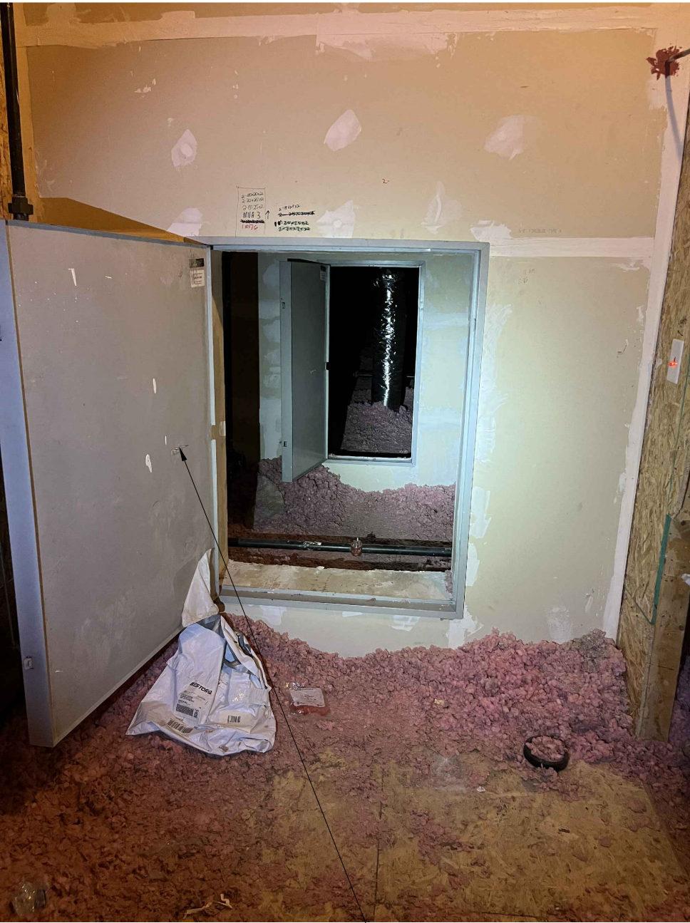
INSTALL SPRING CLOSERS ON ALL ATTIC HATCHES IN RATED FIRE BARRIERS
