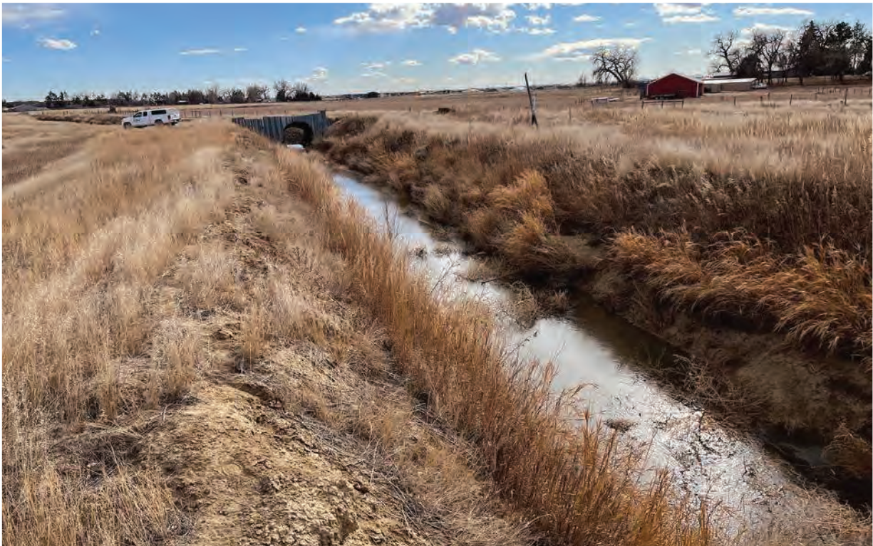
Photo 8 - Overview of the Number 8 Outlet Ditch in the western portion of the project area. View is to the south.
