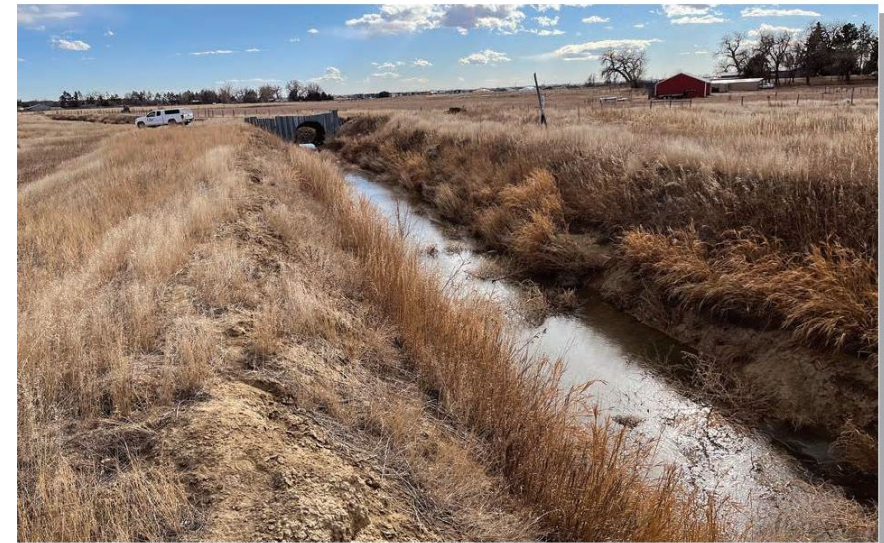
Photo 8 - Overview of the Number 8 Outlet Ditch in the western portion of the project area. View is to the south.
