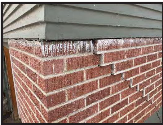
Photo 1: Crack in Foundation at NE Corner
