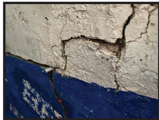
Photo 2: Interior View of Foundation Crack at North Wall Basement Window
