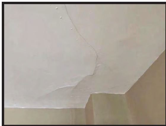
Photo 3: Cracking and Sagging Plaster at Ceiling
