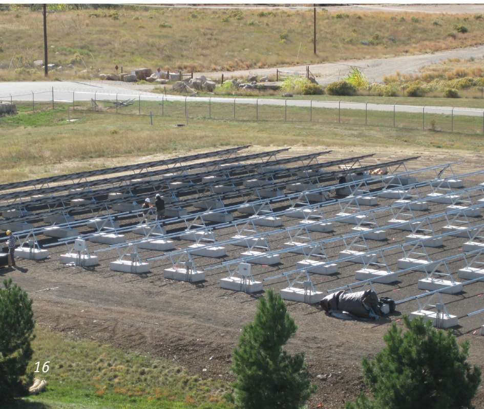
Solar Farm Water Treatment Plant.
