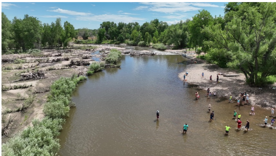
Visitors enjoy the river near the newly constructed award-winning riffle crest diversion structure.
