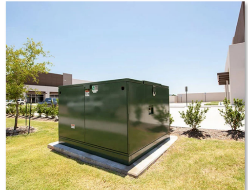
Pad Mounted Switchgear at Drake/Dixon
