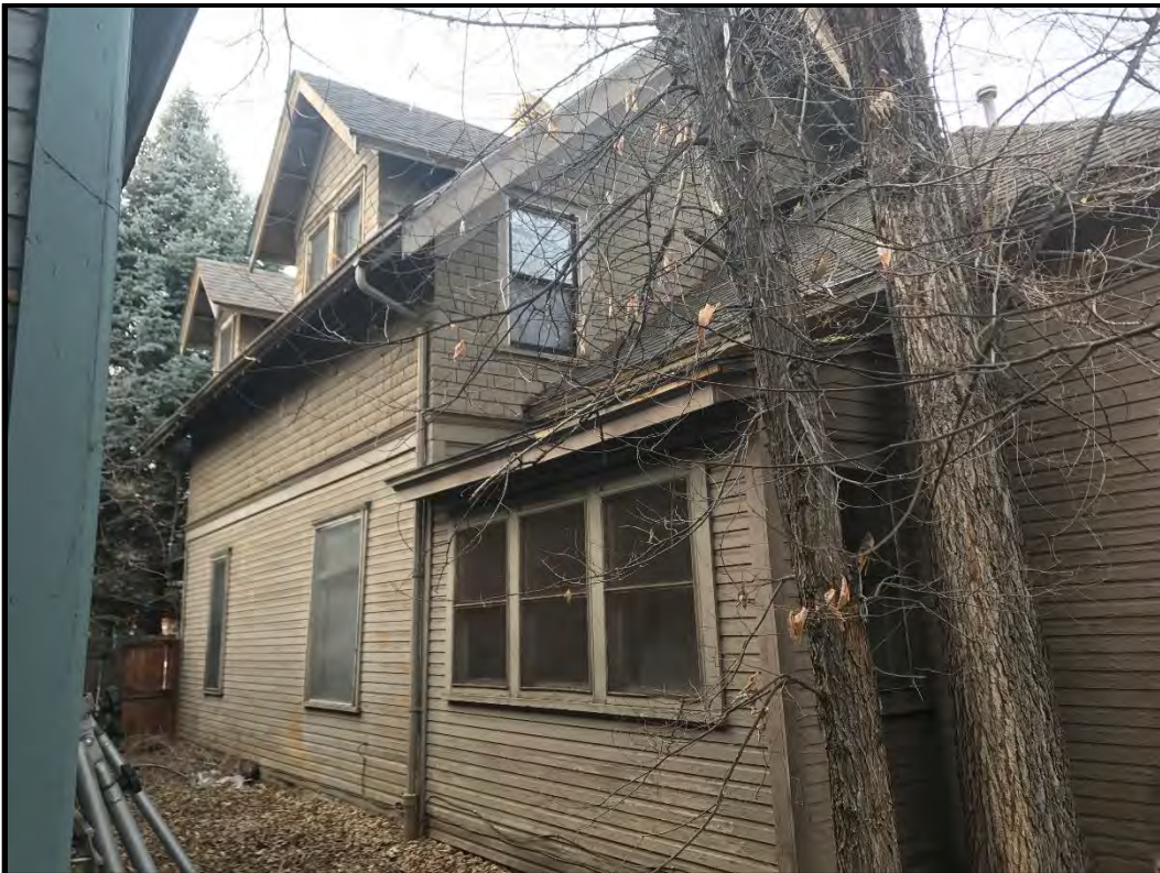
724 South College Avenue, south elevation and small shed-roofed rear porch or mud room, looking NW.
