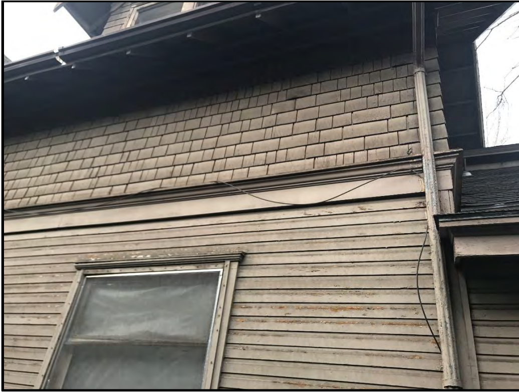
724 South College Avenue, showing wood drop siding (first floor) and shingle-clad upper story walls.
