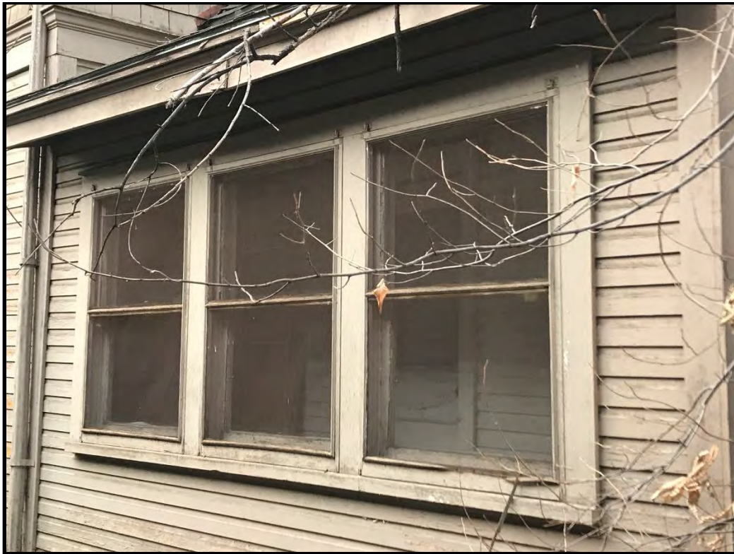
724 South College Avenue, ribbon of windows on south side of small rear porch.
