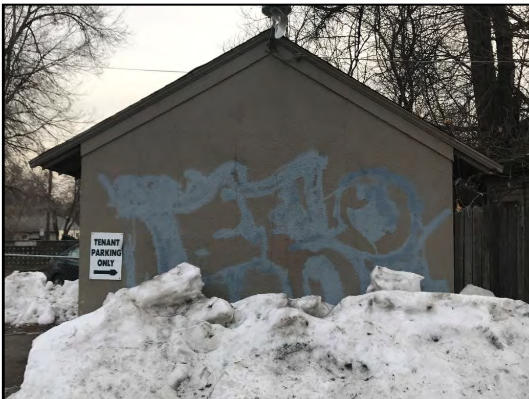
724 South College Avenue, closer view of north elevation of detached garage, looking south.
