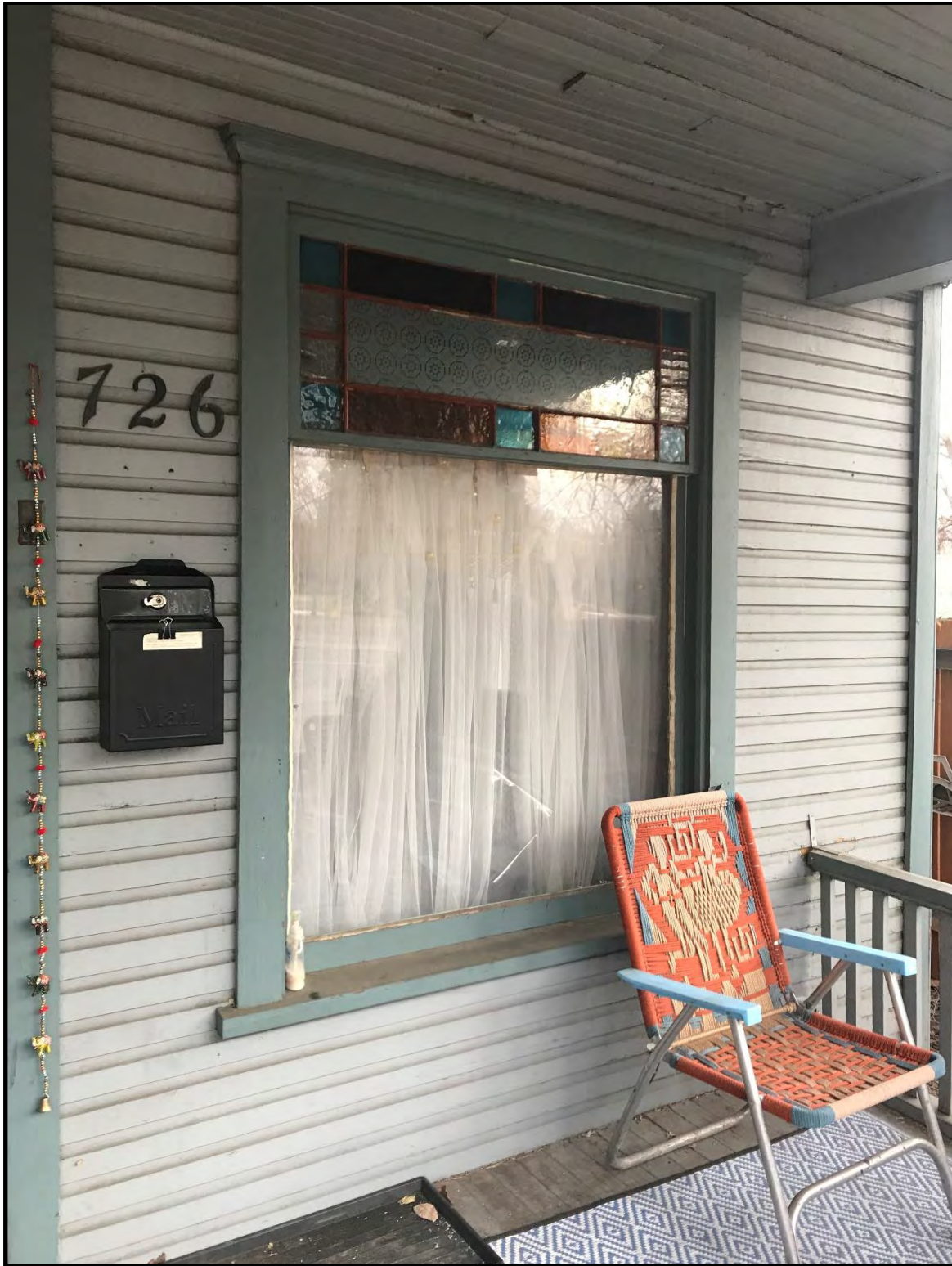
726 South College Avenue, large sash-and-stained glass transom window on façade, looking southeast.
