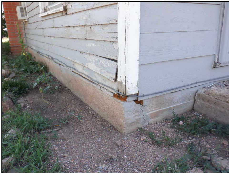
Figure 6: Feature 1, condition of northwest corner (Image #621, RLS 8/23/2022).
