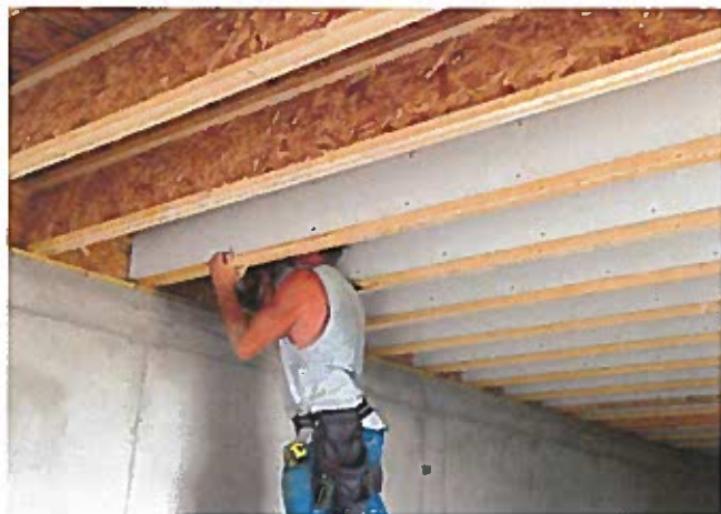
Installing 1/2-inch gypsum board to I-joist webs is one of several methods builders and installers can use to meet the IRC provisions.
