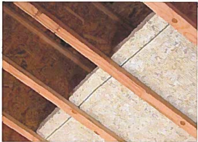
Installing mineral wool between I-joists is one of several methods builders and installers can use to meet the IRC provisions.
