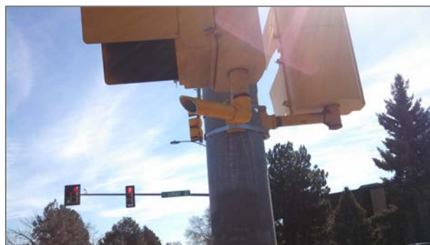
FIGURE 28: THE DETECTION CONFIRMATION LIGHT IS LOCATED BENEATH THE PEDESTRIAN SIGNAL HEAD.
