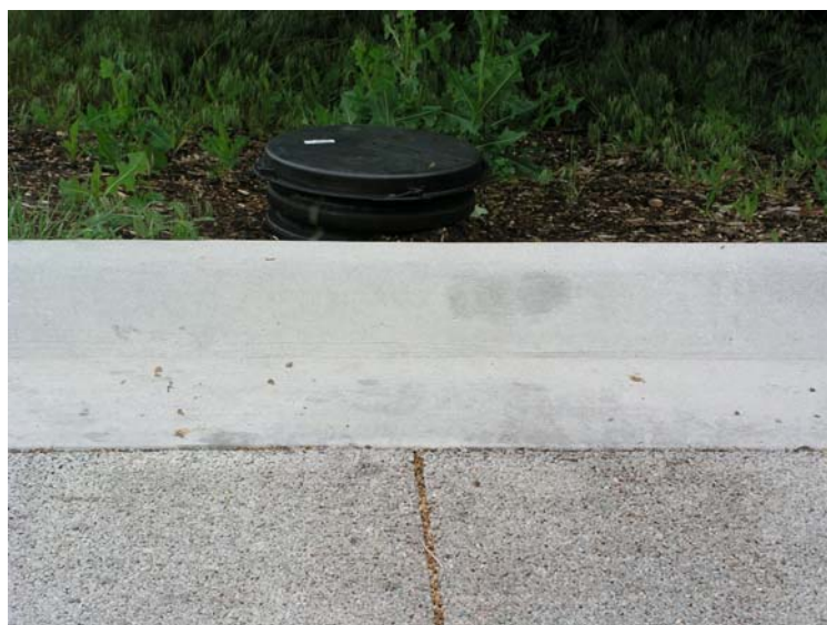
Monitoring vault at CTL Thompson site
