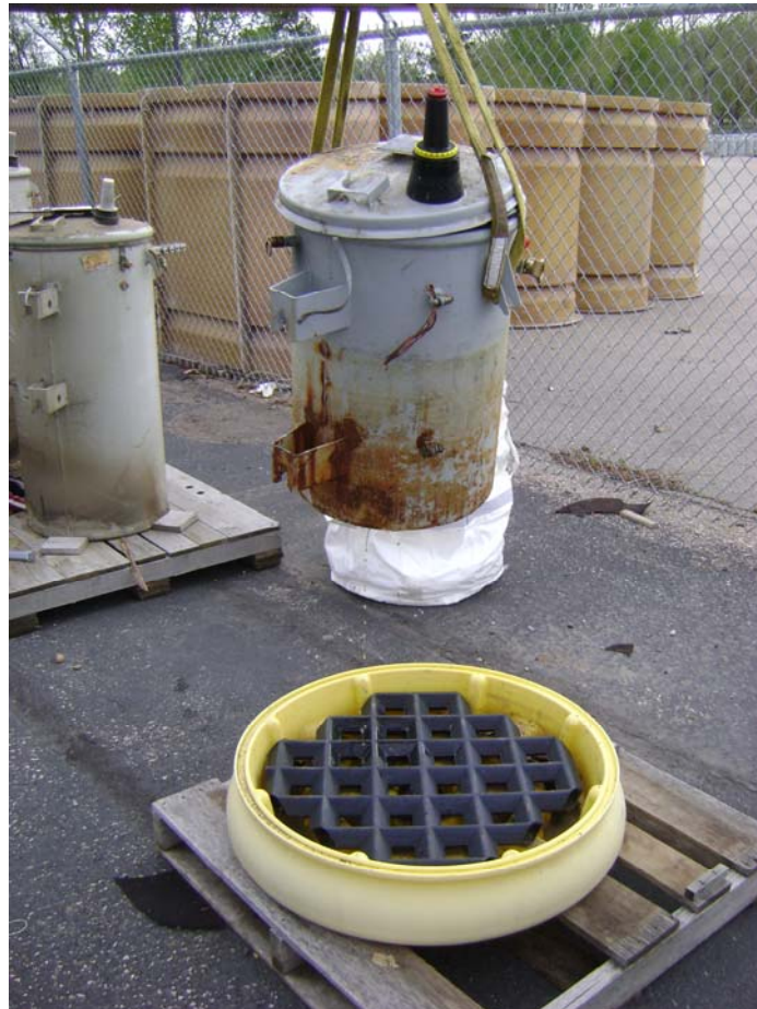
Leaking electrical transformer spill containment.
