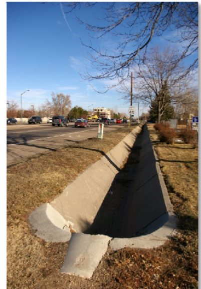
The concrete-lined ditch on the south side of Harmony Road, just east of College Avenue.
