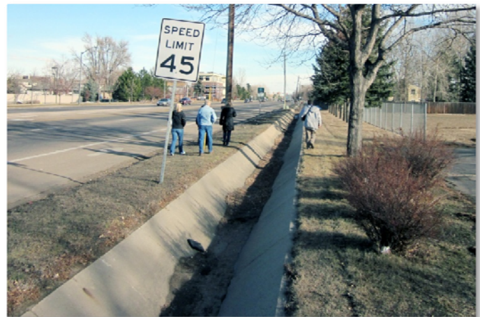
Concrete-lined drainage ditch creates a barrier for transit rides.
