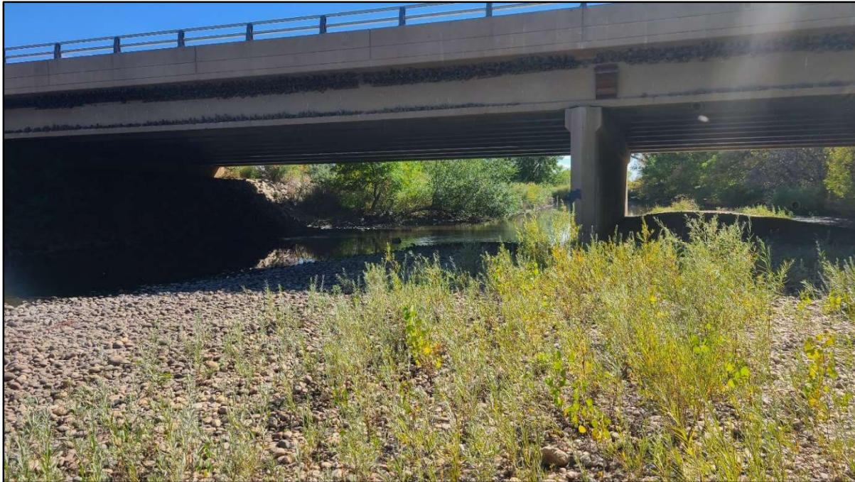
Photo 1. Prospect Corridor Improvements: Facing south, Cache la Poudre River flowing beneath Prospect Road bridge. Evidence of bird and bat habitat was seen on the bridge. East riparian corridor was steep and heavily vegetated.
