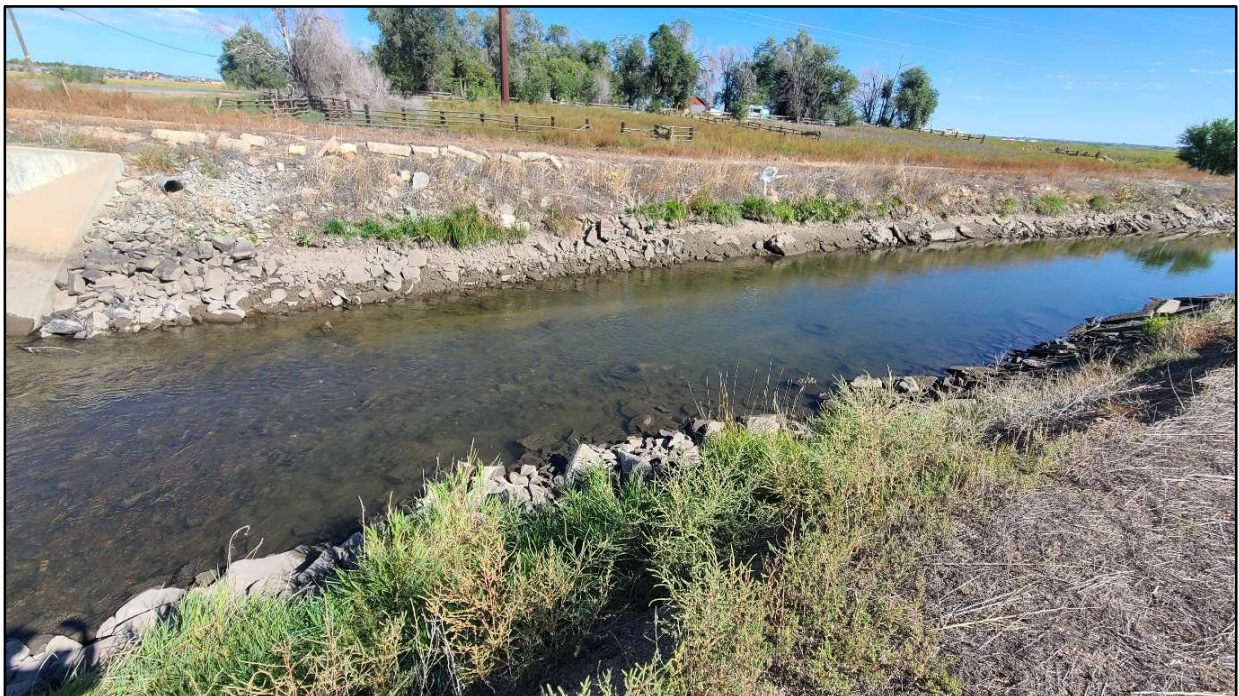
Photo 12. Timberline Road North – Segment 2: East side of Timberline Road (Segment 2) at the crossing of the Larimer and Weld Canal. Canal had steep banks and was armored with riprap. Vegetation was relatively sparse.
