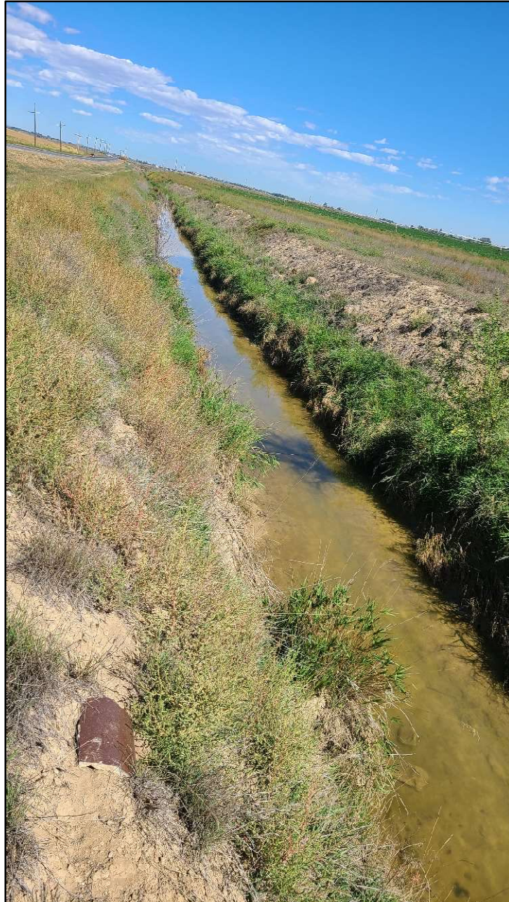
Photo 13. Timberline Road North – Segment 2: Facing north, the Number 8 Canal, parallel to Timberline Road (segment 2). Channel had steep vegetated banks which were eroding in areas. The canal continues south where it eventually drains into the Larimer and Weld Canal.
