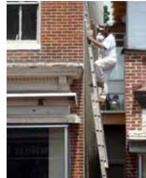
If a feature is deteriorated or damaged, repair it to its historic condition.
