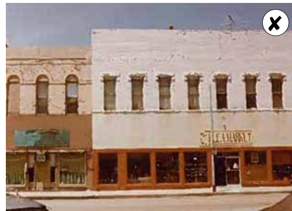
Interim image of missing cornice.
