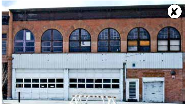
Before rehabilitation: upper story windows in need of repair.
