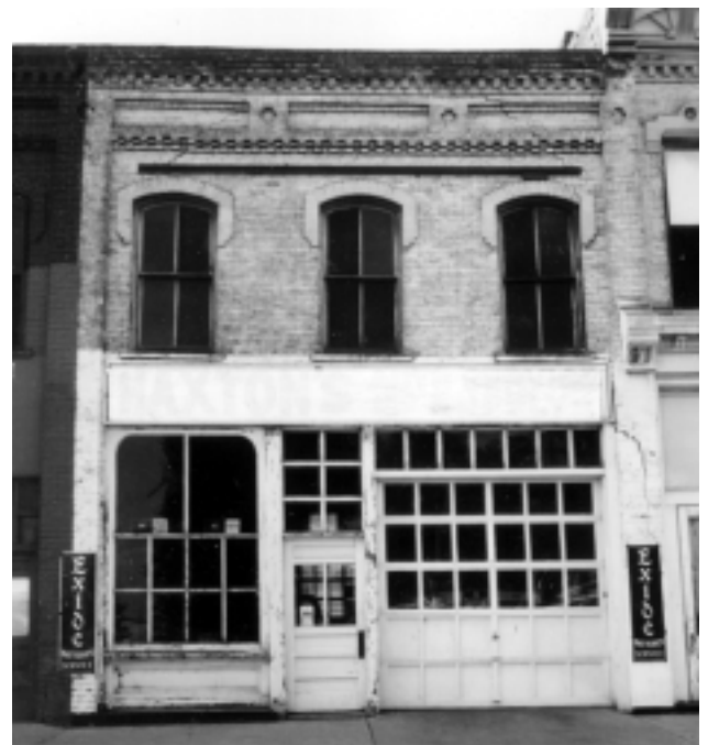
Where the brick has been painted, it is usually best to leave it that way and simply repaint when a fresh look is desired.
