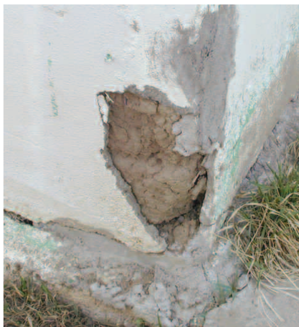
Figure 6. Adobe bricks show through a crack in the stucco of this Alta Vista house. (Photo by the author.)
