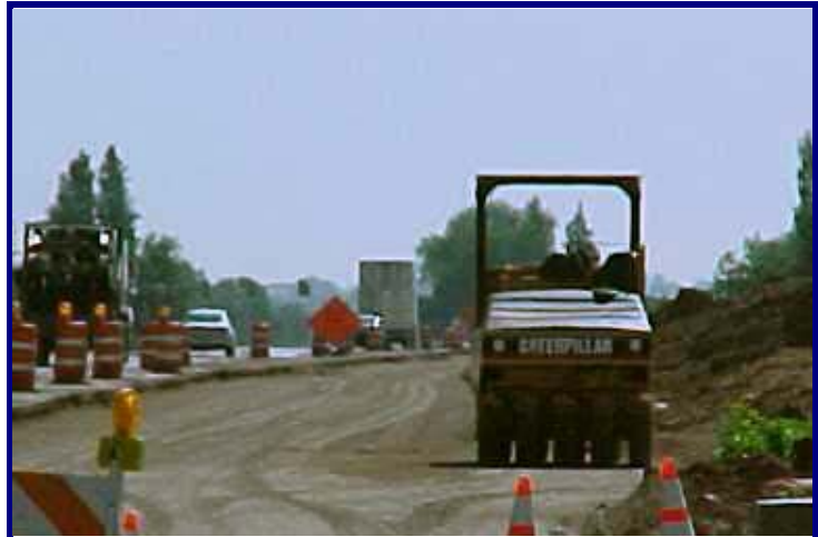
FIGURE 1: The widening of Harmony Road (shown above) was funded through the Street Oversizing Program and developer participation.
