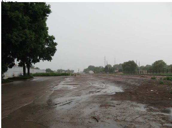
Construction of the BRT will create new opportunities for the "backside" of West College Avenue properties.
